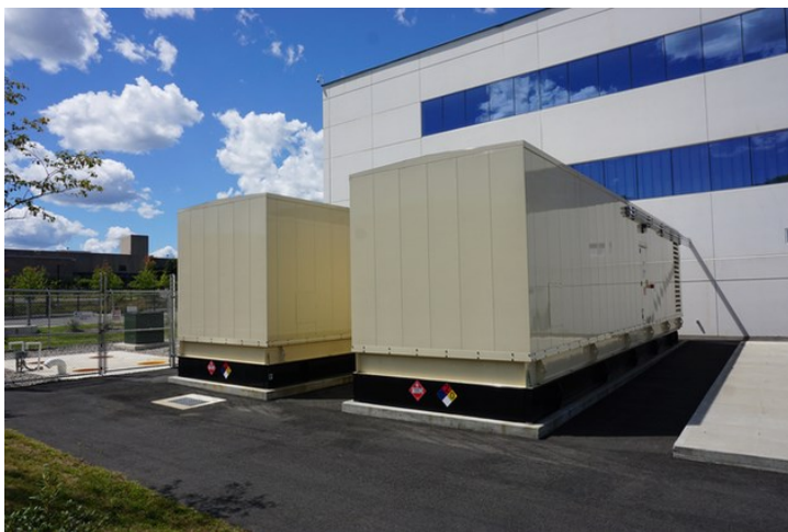
Diesel-powered back-up generators at the 168,000 square foot Norwalk data center.
