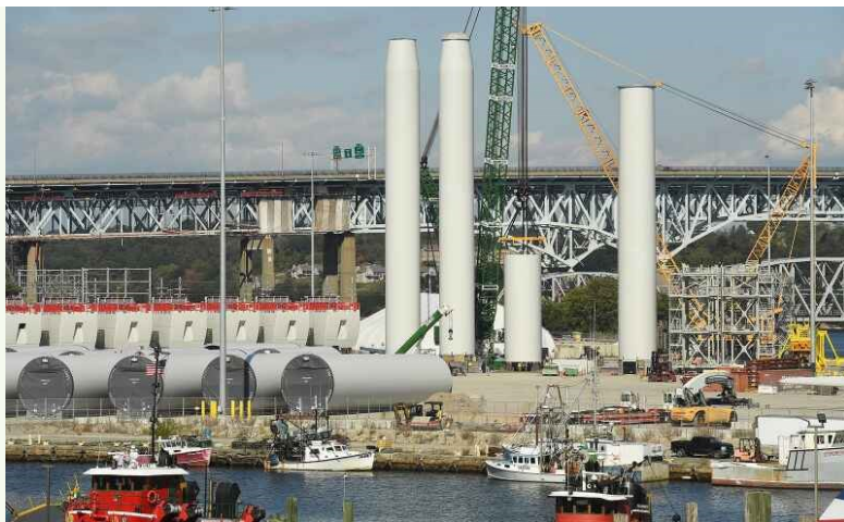
A familiar view from Gold Star bridge! Wind turbine tower sections being put in place last October at New London's State Pier in preparation for Ørsted's South Fork Wind Farm project off the coast of Long Island, N.Y. The towers will rise 518 feet above the surface of the water when installed. Photo credit: Dana Jensen, The Day
